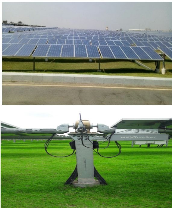
Fig. 2: Solar PV array configuration and SAT
