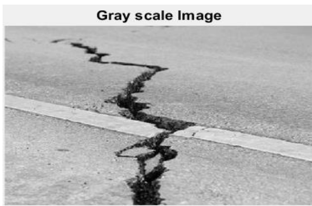
Figure 3 Gray scale of longitudinal crack image
