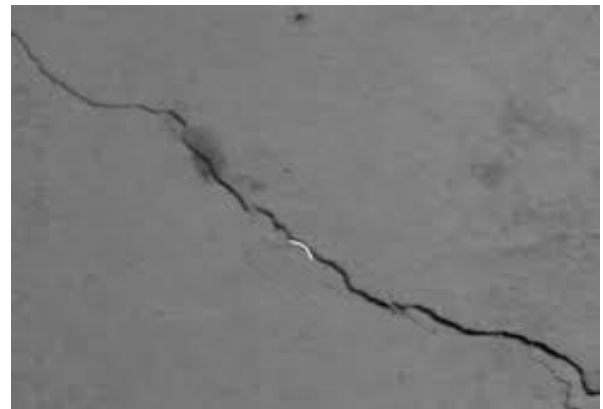
Figure 9 Original of transverse crack image
