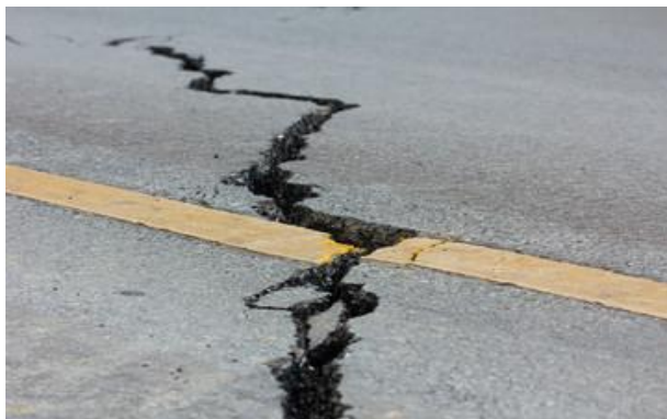
Figure 2 Original of longitudinal crack image
