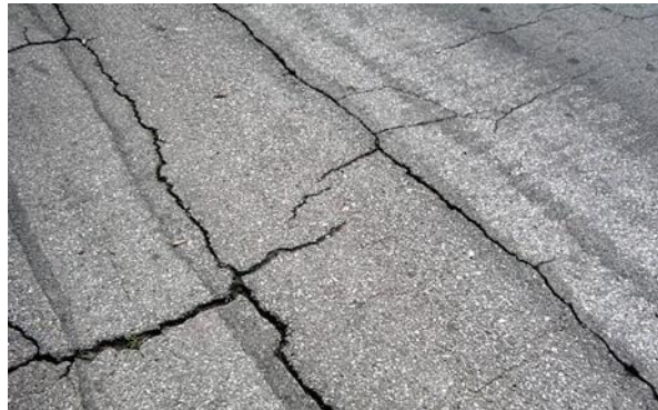
Figure 23 Original of block crack image
