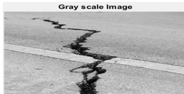
Figure 2 Original of longitudinal crack image
