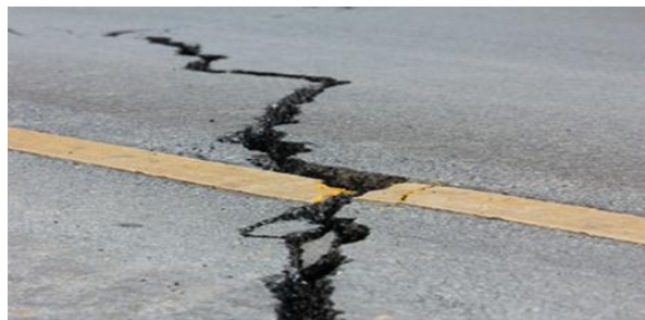
Figure 3 Gray scale of longitudinal crack image
