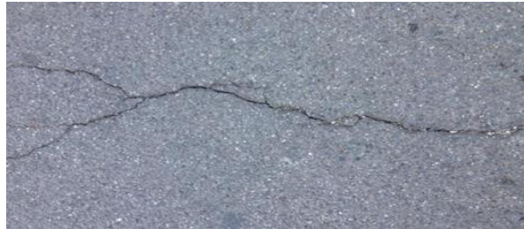
Figure 16 Original of alligator crack image
