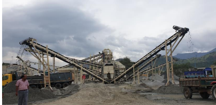
Aggregate crushing unit
