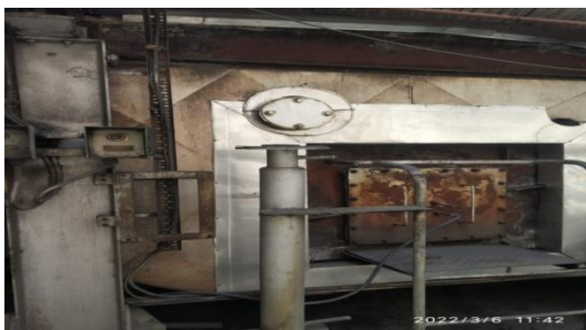
Fig 1(b) -Tapping point taken for Flue gas Acquisition
