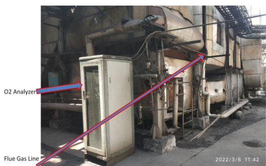
Fig 1 (c) O 2 analyzer Probe monitoring Control Panel
