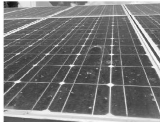
Fig.5. Degraded PV module status
