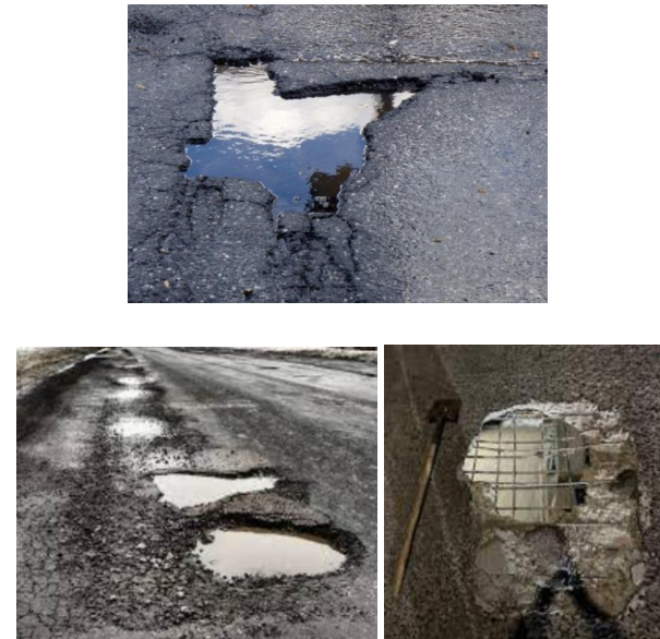
Figure 1: Examples of potholes
