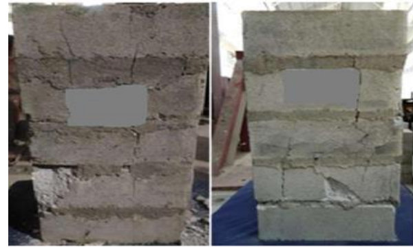
Fig.11 (a) 1:6 masonry specimens with numerous cracks and (b) Failure resulted from a single crack in 1:3) masonry specimens.
