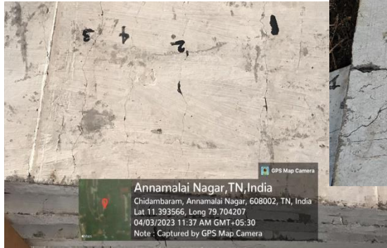
Fig.15. Crack pattern of GPC-Steel Slab
