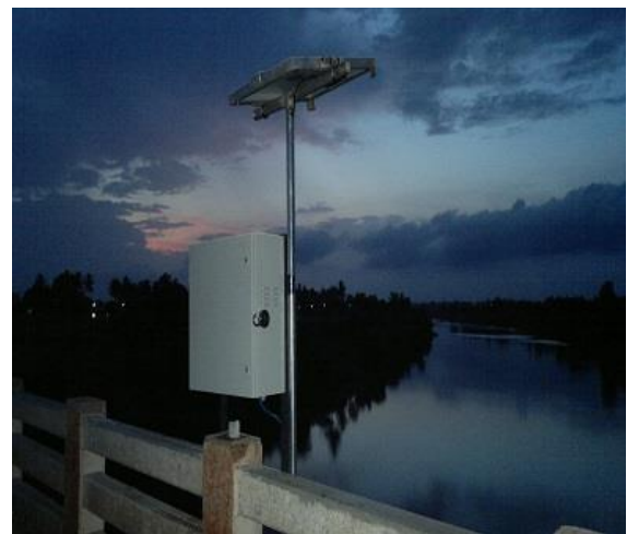
Figure 2. Flood Monitoring System with IoT Sensor RTDS.
