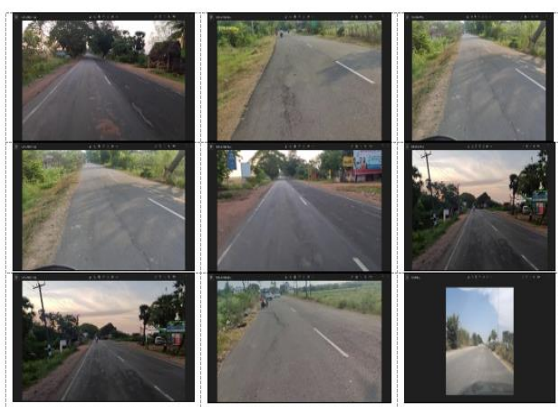
Figure 1. State Highway Road Damage Dataset Sample.
